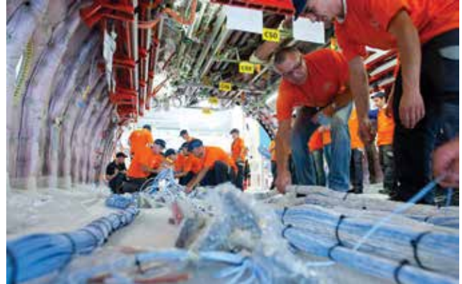
With CATIA, Airbus implemented a full 3D Master approach to design the electrical harness installation for the A350 XWB. Any errors were corrected digitally before physical installation. (Photo © 2013 Airbus SAS / F.Lépissier)
